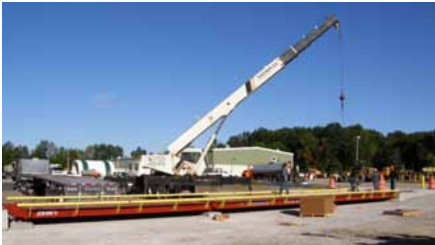
Figure 3 shows the scale being placed on the concrete foundation. The approaches to the scale were also prepared before the scale was installed.
