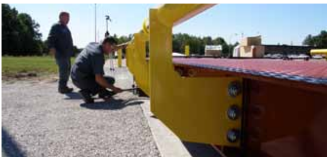
Figure 1 show technicians from the Youngstown, Ohio Brechbuhler branch grounding the truck scale. This scale is impervious to lightning strikes.
