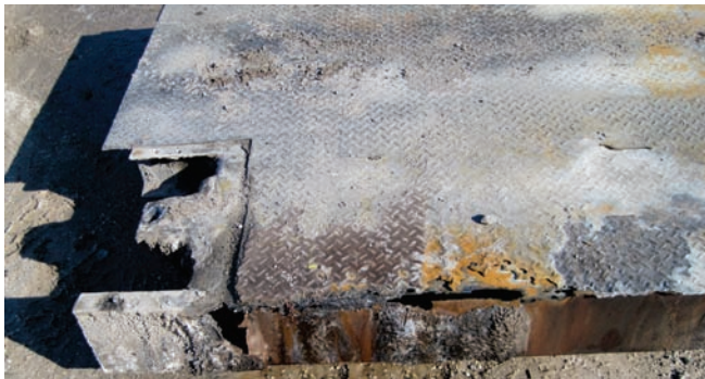
Figure 4 of existing scale condition
